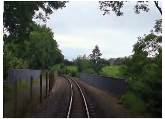
Figure 8-27 – Topside Bontnewydd Viaduct Obstruction - CD-03-04
