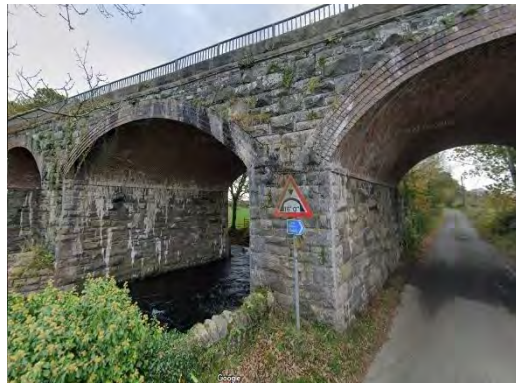
Figure 8-26 – Underside Bontnewydd Viaduct Obstruction - CD-03-04
