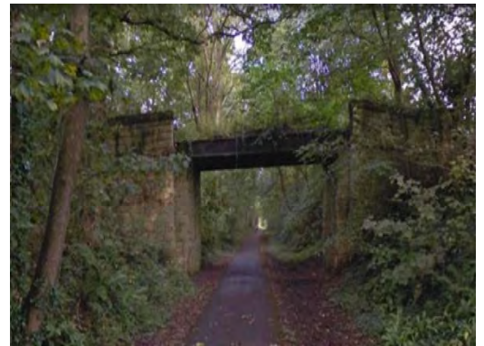
Figure 7-45 – Road crosses alignment Obstruction BC-09-03
