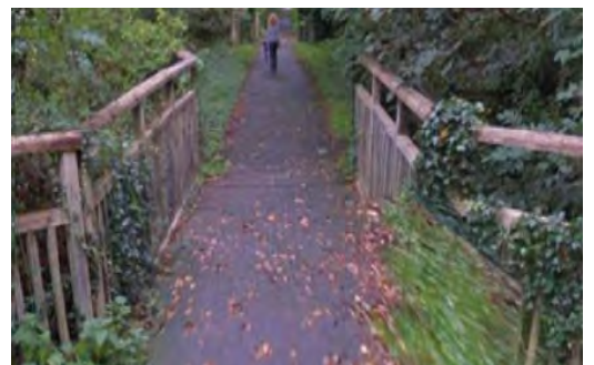
Figure 7-47 – 2 Timber Underbridges Obstruction BC-10-01
