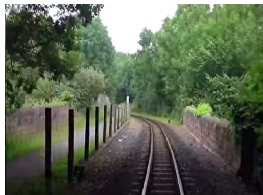
Figure 8-15 – River Seiont Underbridge Obstruction - CD-01-07
