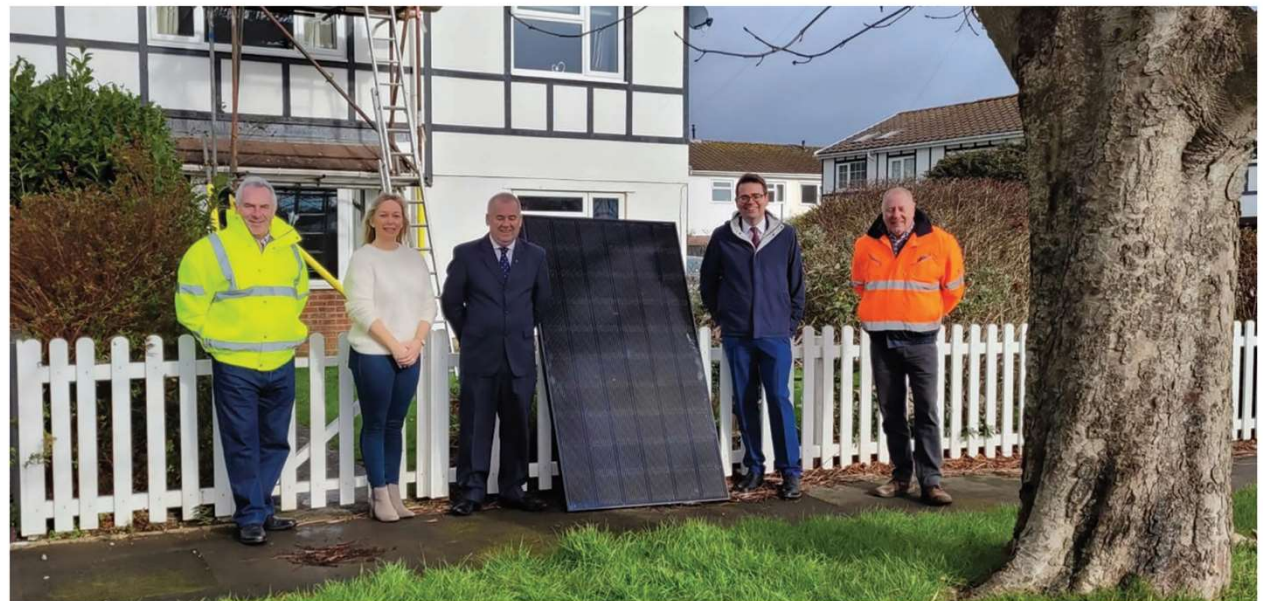
Challoch Energy and NuVision Energy team with local councillor and resident of South Cornelly during home installation of solar panels.
