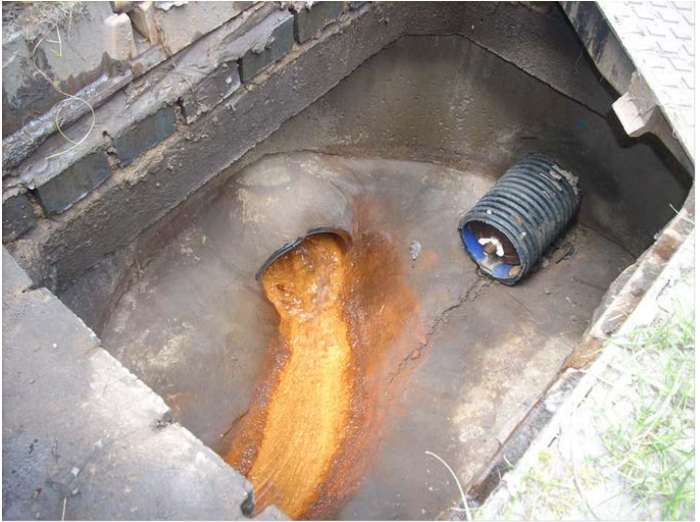
Figure 5.2. Tan y Garn discharge manhole chamber
