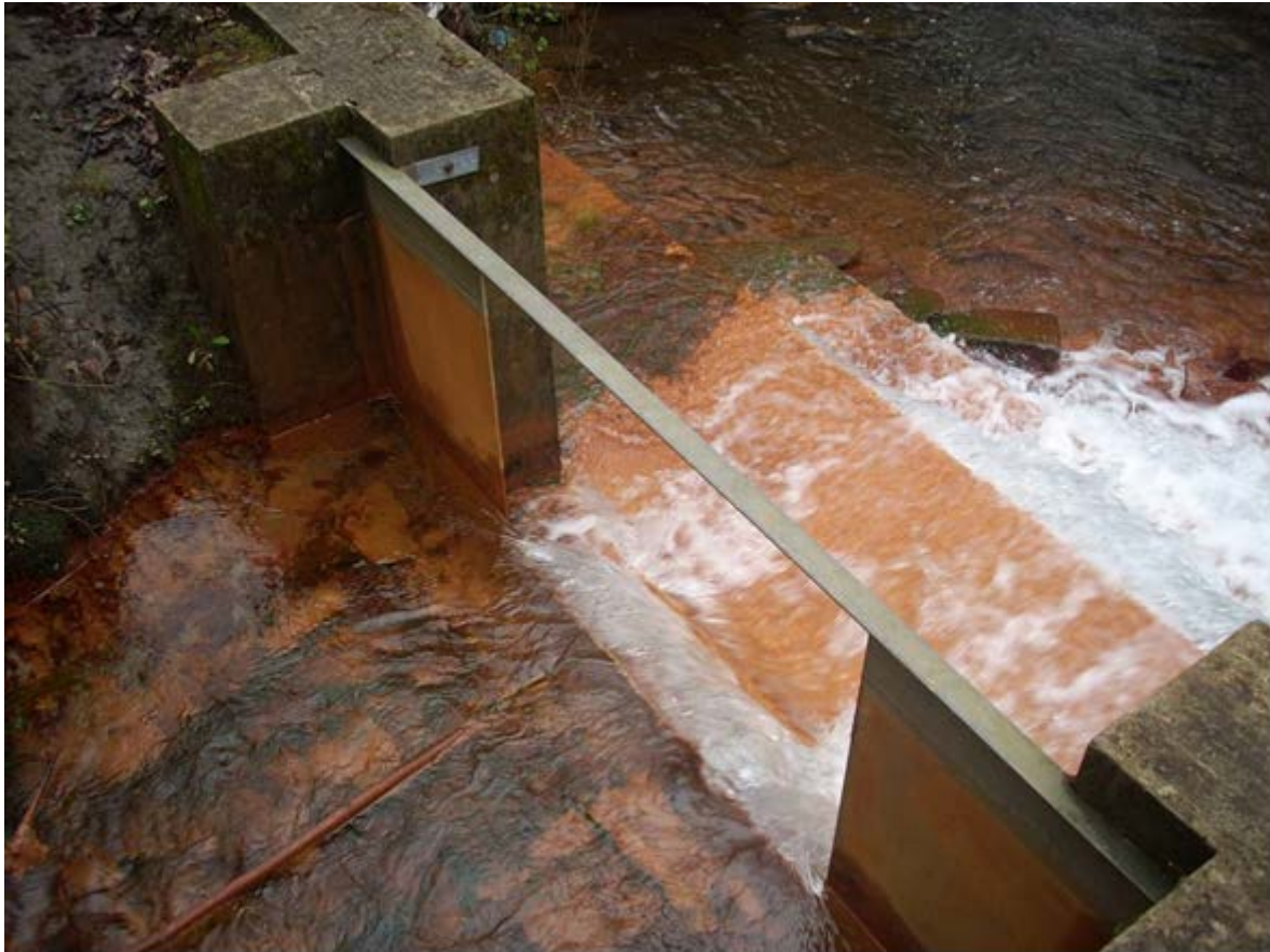
Figure 5.2: Cefn Hengoed No1 (main) Discharge
