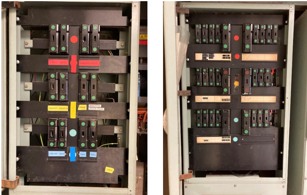
Typical Ward Riser essential and non-essential Distribution Board
