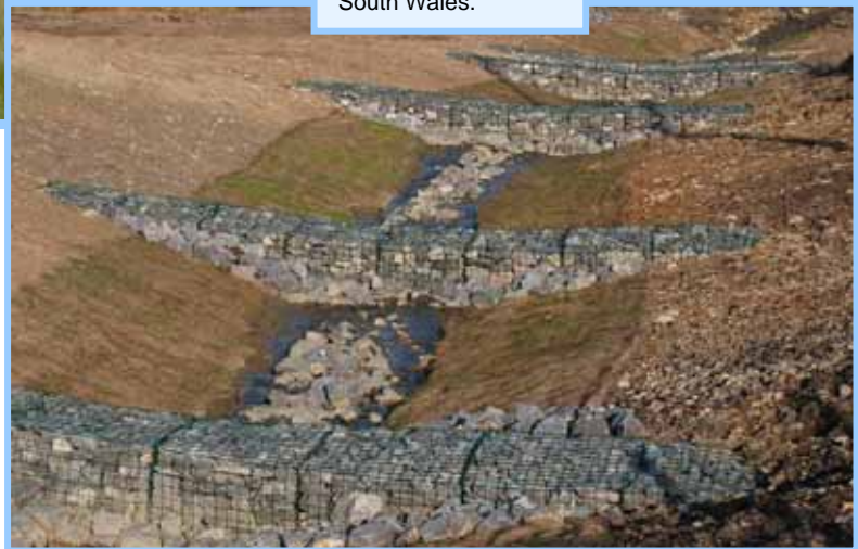
Examples of erosion control schemes at opencast coal sites in South Wales.
