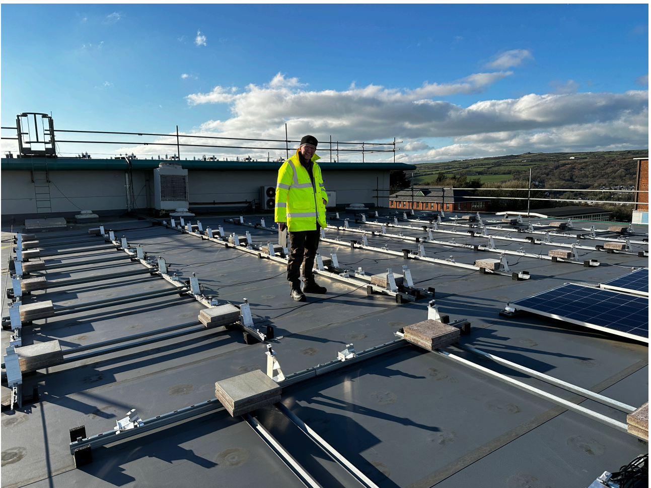
Solar photovoltaic (PV) panels, Egni Co-op
