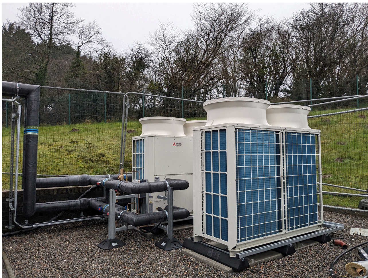
Carmarthenshire County Council, heat pumps for schools
