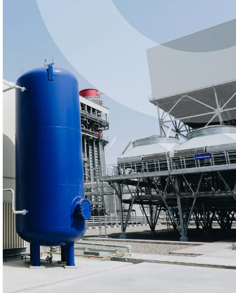
Power plant tankers and cylinders for oxygen, hydrogen and water storing.
