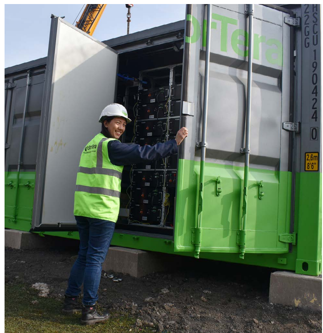
StorTera batteries in shipping containers to store solar energy generated on site.
