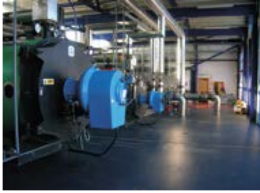
Back up oil fired boilers in boiler station Reproduced with permission of SHEaP
