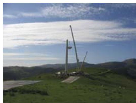
Installation of second community wind turbine in 2003 Reproduced: Need approval from CAT, media@cat.or.guk
